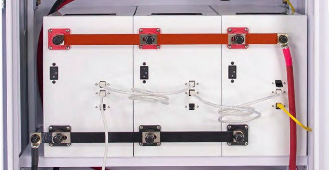
Figure 8.0 – AmpliPHI Wiring using Interconnecting Busbars
