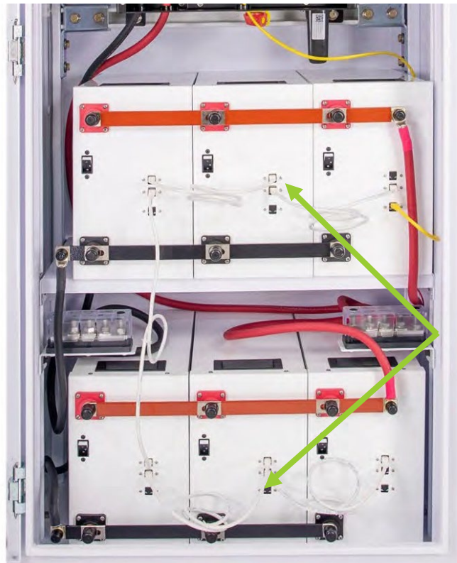
Figure 12.0 – AmpliPHI Batteries Networked
